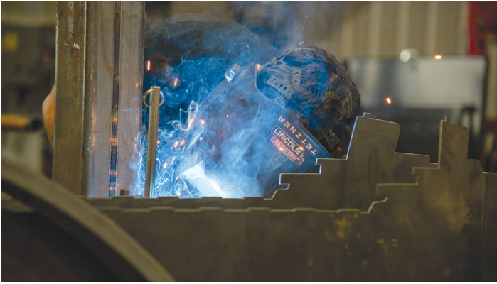
Matt Tetzner adds welds to the hardware he fabricated to mount the weathervane on its tower.
